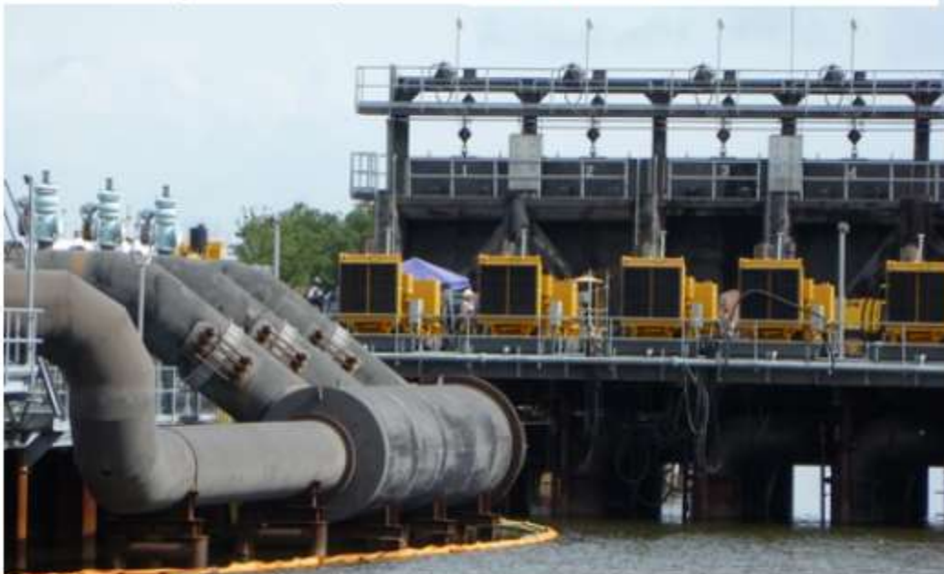
New floodgates at the 17th Street Canal (Photo by Betty Ann Bowser)
